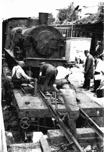
Jacking up the boiler unit, so that the leading unit can be rolled under it.
