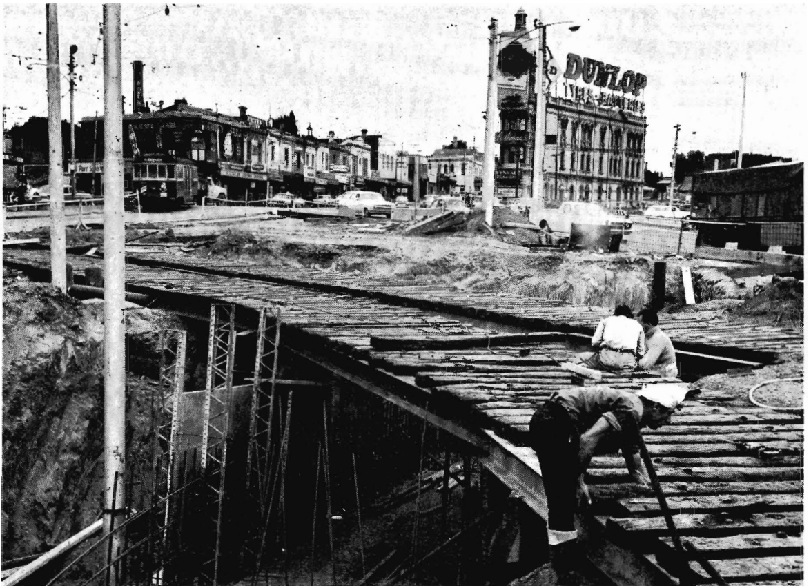
Work in progress at St. Kilda Junction on which $12 million will be spent. As a result, it has been estimated that vehicles carrying about 4,800 more people will be able to enter the city through this gateway. The additional cost is $2,500 per person. For $5½ million spent on the Box Hill group of railway lines, facilities could be provided for trains carrying an extra 22,000 passengers. This gives an outlay per head of about $250—that is one-tenth of the outlay per person at St. Kilda Junction.
