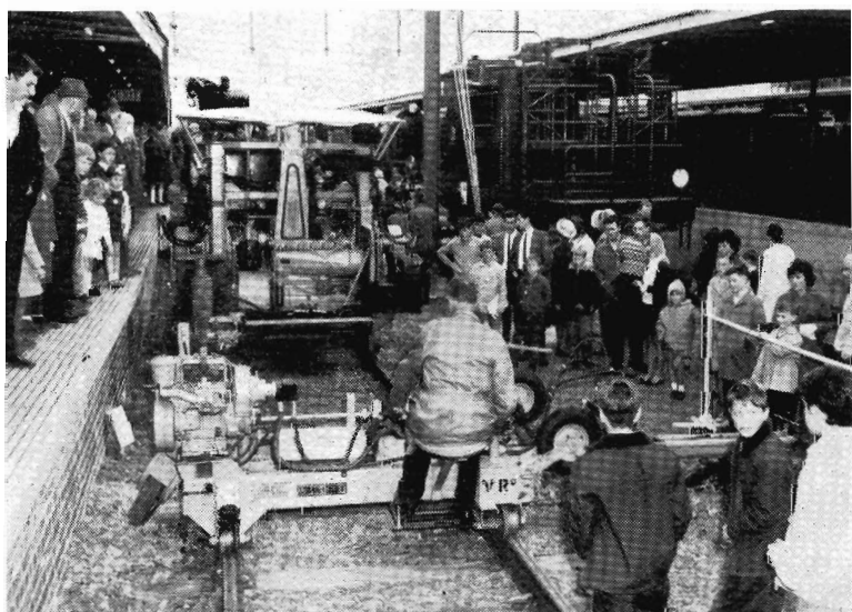
Crowd watches Aresco sleeper renewer (in foreground) and Plasser tamping machine. In right background is the clearance van.
