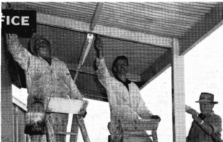
Painting Foster railway station are (from left) Painters R. Gardiner, A. Richards, and Leading Hand Painter L. Hart.
